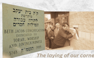
The laying of our cornerstone, 1988, photo from the Upper Midwest Jewish Archives
